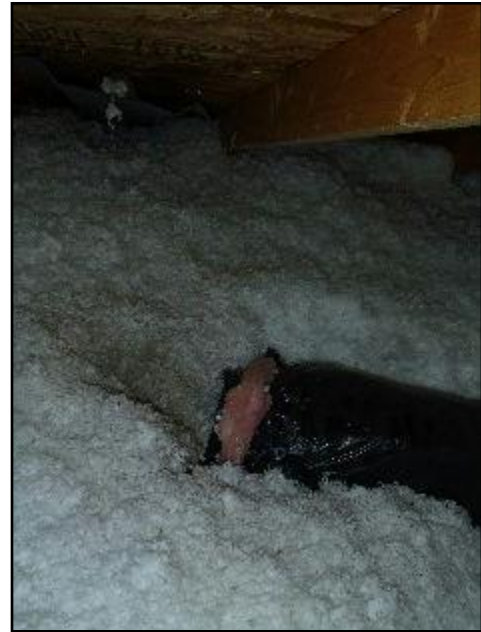
111. Not vented to exterior
