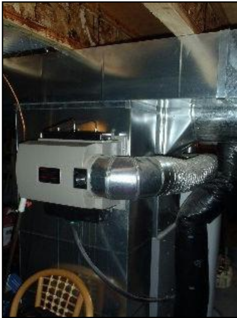
64. Duct mounted bypass humidifer
