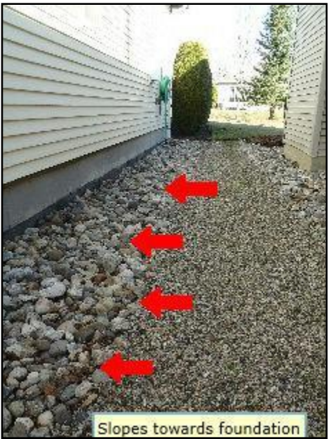
28. Improper slope or drainage
