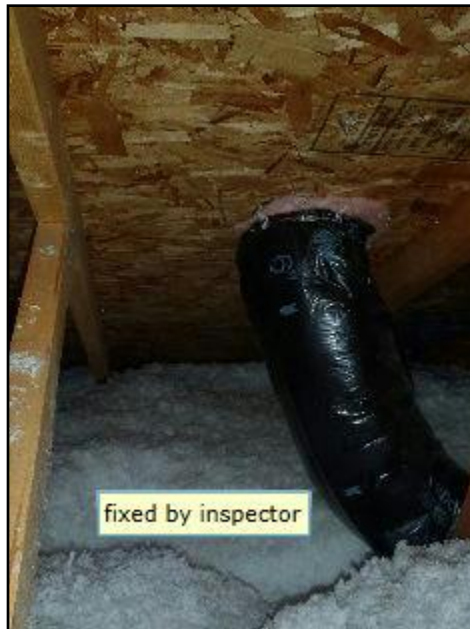
112. Not vented to exterior
