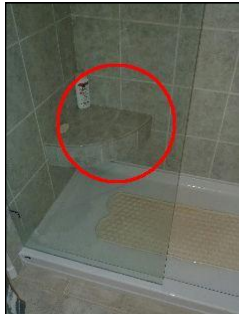
80. Caulking loose, missing or deteriorated
