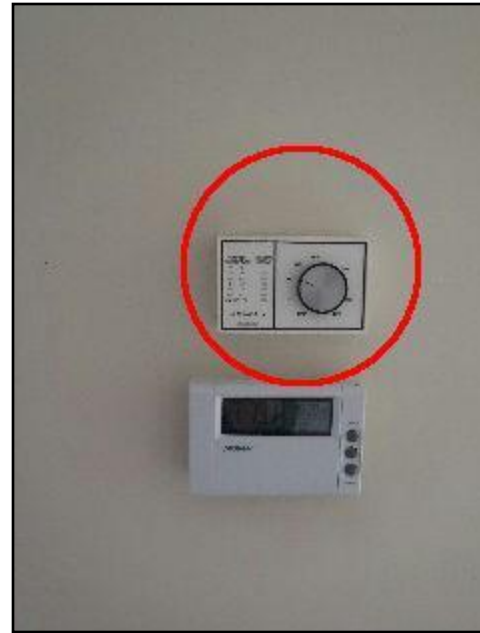
65. Duct mounted bypass humidifer
