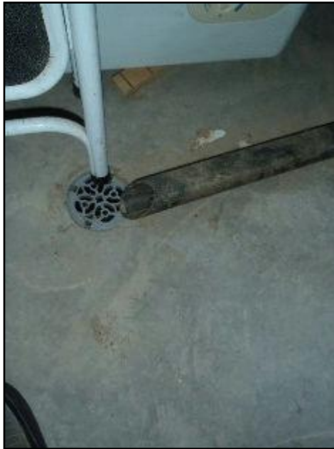
77. Near water heater
