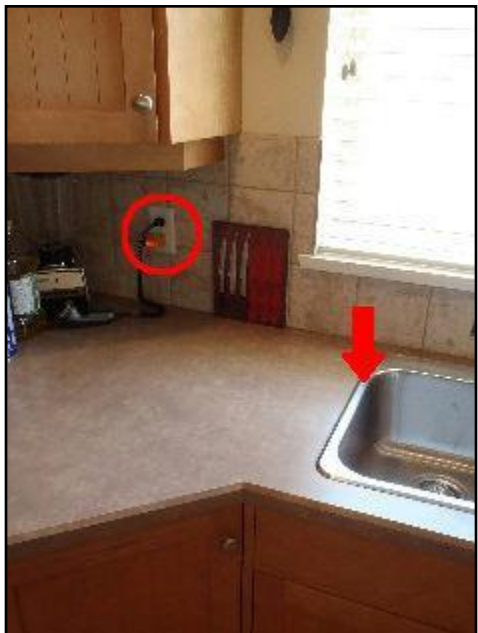
53. Ground Fault Interrupter (GFI) needed
