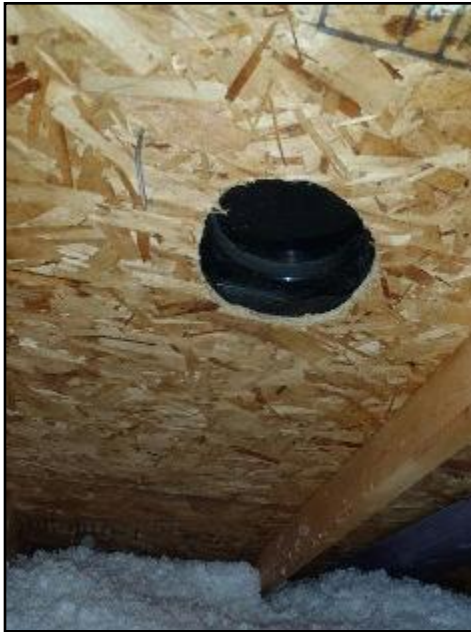
110. Not vented to exterior
