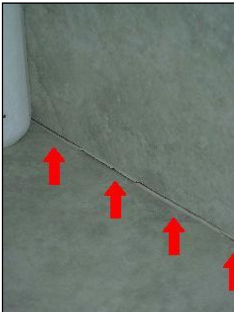
79. Caulking loose, missing or deteriorated
